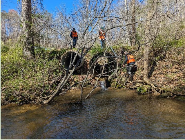
Culverts that empty into Mill Creek near Reynolds Mill. Photo by Anna Wheeler.
